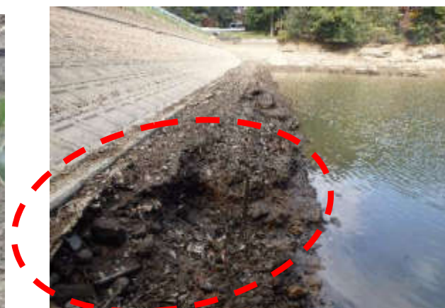
②堤体上流法面の浸食
