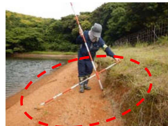
②堤体上流法面の浸食
